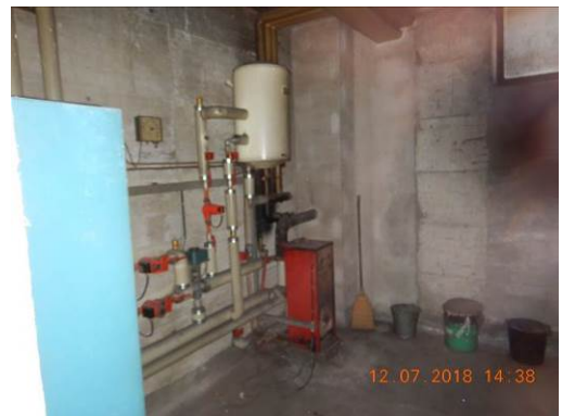
Locale caldaia – Piano interrato
