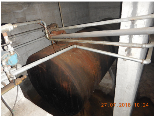
Distributore gasolio – Diesel Tankstelle „A2.2“ Serbatoio – Tank 1
