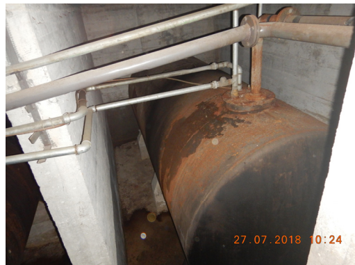
Distributore gasolio – Diesel Tankstelle „A2.2“ Serbatoio – Tank 2
